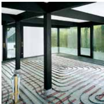
Underfloor heating living area
