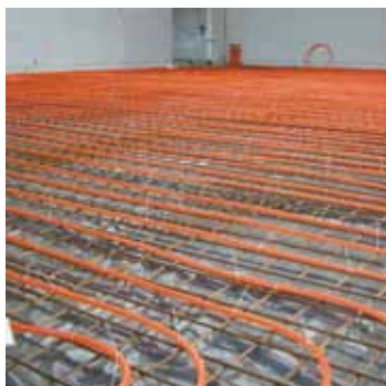
Industrial floor heating
