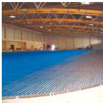
Chilled area, ice stadium
